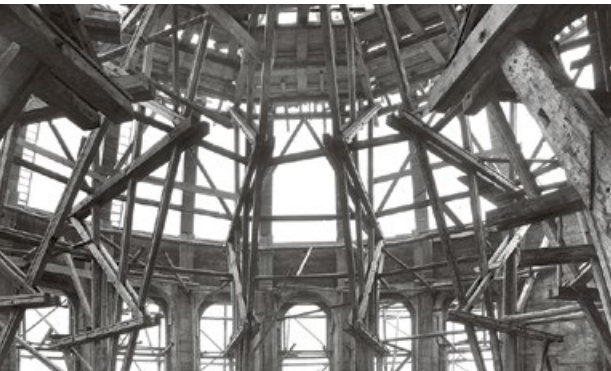
The building of the ETH dome in 1919/20 was both a reflection of the past and an indication of growing self-confidence.
